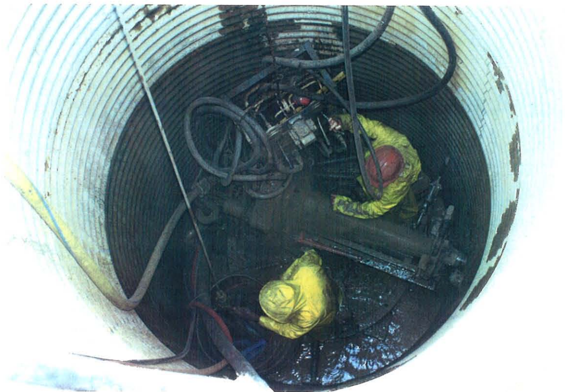
Figure 21. Drilling lateral into water bearing unconsolidated materials. Note drilling crew must wear water proofs and safety glasses during this operation.
