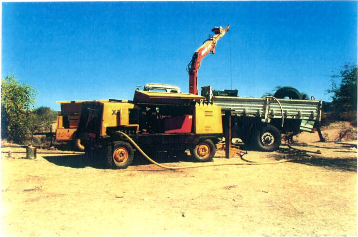
Figure 16. Large capacity Atlas Copco 350 l/sec, 20 bar compressor, used to supply compressed air for drilling and jetting in pipe.
