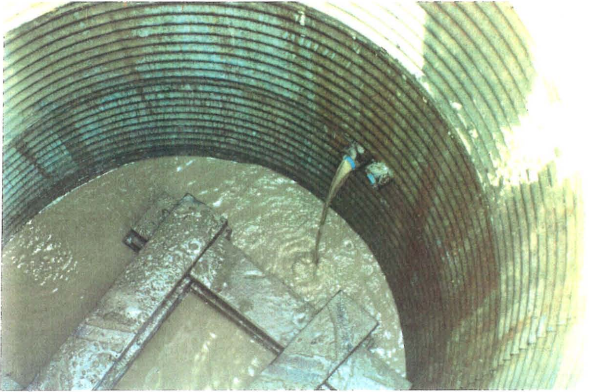
Figure 49. Water flow from second lateral heavily charged with silt, Matshelagabedi.
