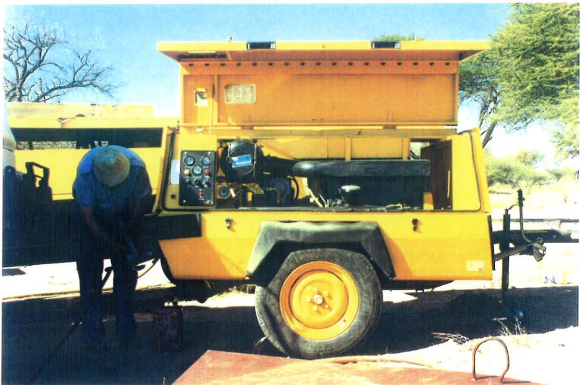
Figure 17. Small capacity 110 lb/in 2 , 125 cfm compressor, used to supply air for dewatering pump operation.
