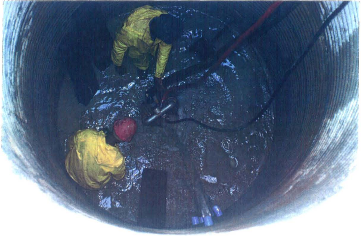
Figure 36. Flowing laterals within the completed Gulubane collector well.
