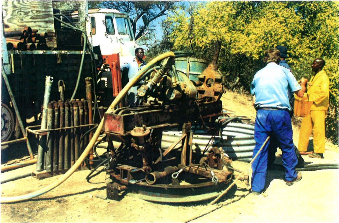
Figure 14. Horizontally mounted Hydroquest 2 rig on circular base plate with jacks for mounting within a 2 m diameter well-shaft. Note cradle with drill rods and drilling bits to left of rig.
