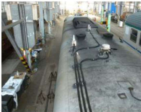
Fig. 2. Antennas placed in ALN 668 3114 roof (Courtesy of ASTS).
