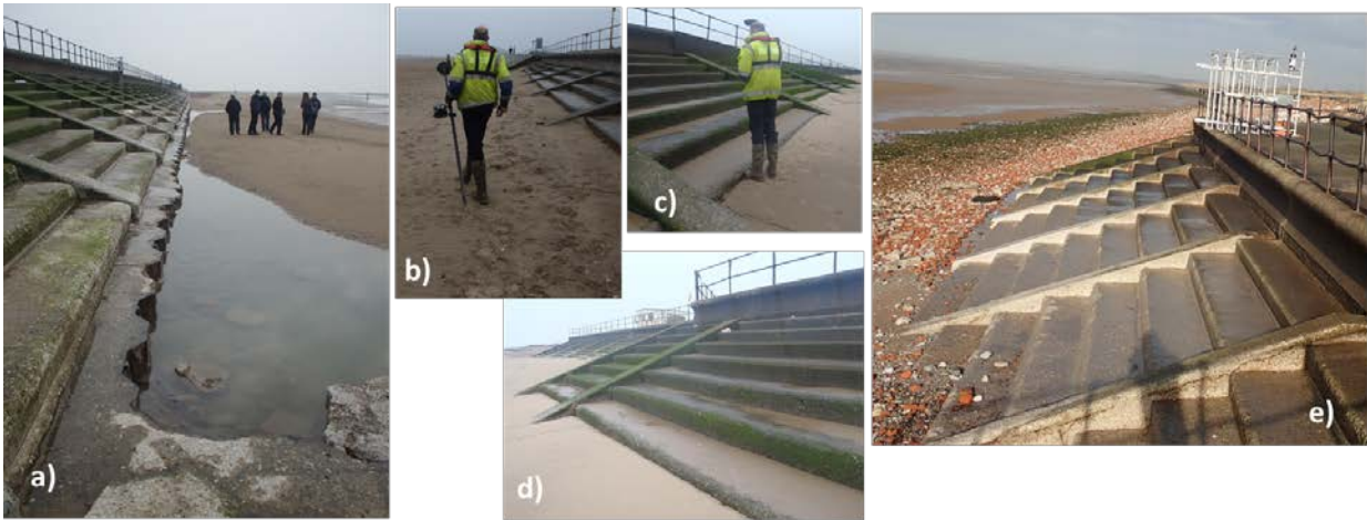
Figure 4.40: a) Looking south from the bottom of the slipway along the Crosby sea wall 17 th March 2015. The beach level during a SC survey 13 th April 2018 a) just south of the slipway b) seaward of the slipway and c) at the slipway looking north. c) The beach level prior to high water on the 25 th January 2019 with the sheet piling just exposed in front of the 3 most northern stepped revetment sections.
