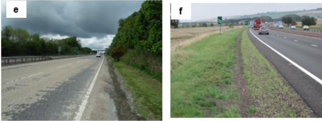
37 38 Figure 1 | clogged HFDs due to: (a) surface cake-layer, (b) pine needles, (c) vehicle over-run, (d) 39 litter accumulation, (e) wear-and-tear of the High Friction Surface Course, (f) vegetation intrusion.
