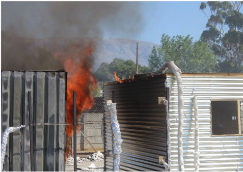
(a) Flames emerging from ISD2 and igniting an exposed timber piece of ISD2
