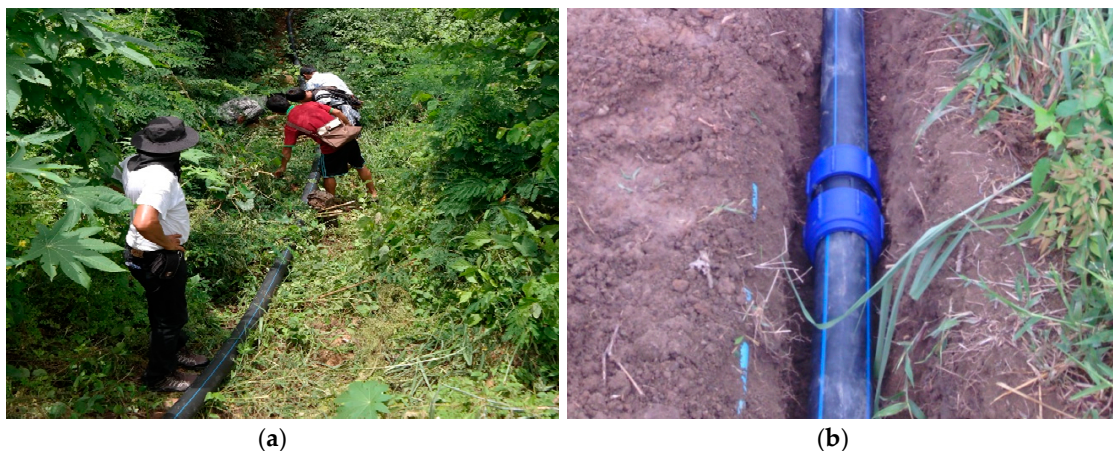
Figure 8. Installation of pipelines (a) and coupling system for the high-density polyethylene (HDPE) pipe connection (b) (photos by the authors): (a) installation of pipeline work; (b) coupling system for HDPE pipeline.
