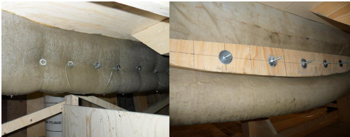
Figure 6 Internal restraints in fabric formwork using discrete ties or continuous web formers
