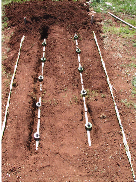
Figure 7.2: Placement of targets before their burial for maximum detection height measurements. The boards help to control the depth of the targets.
