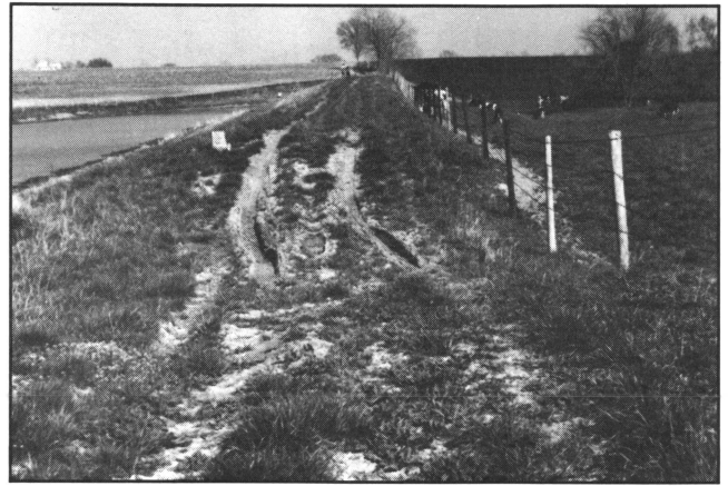
Figure 8. Keep livestock fenced away from the dam and the emergency spillway to maintain a vigorous vegetative cover for erosion control.
