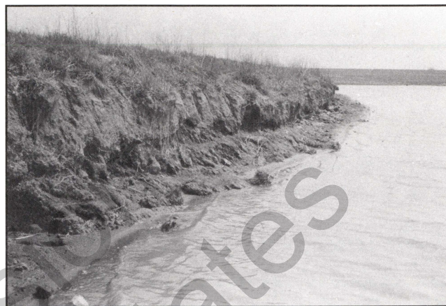
Figure 1. Wave action can cause excessive erosion to the face of the dam.
