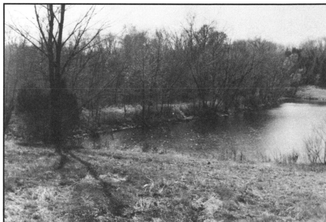
Figure 5. Don't allow trees and brush to grow on the dam or in the emergency spillway.
