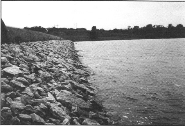
Figure 3. Rock rip-rap may be required to protect a dam from wave action, especially if the dam faces the prevailing wind or has a large pool.
