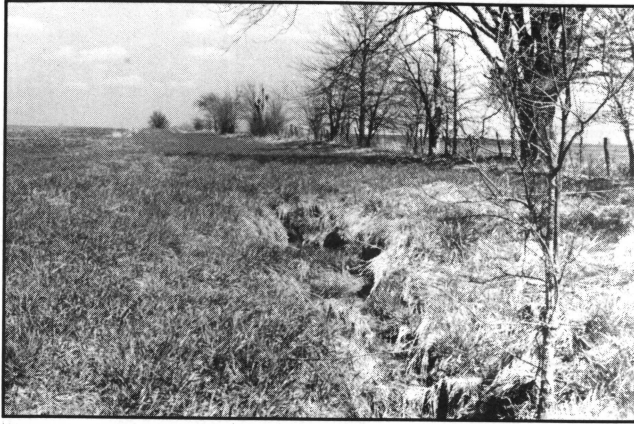
Brush and trees should not be allowed to compete with grass in the waterway. This unstable outlet may require regrading or a grade stabilization structure to eliminate erosion at the lower end of the waterway.
