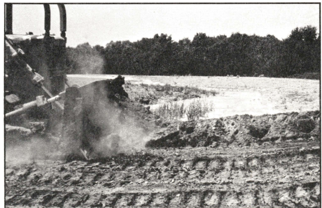
Extremely erosive storms may necessitate removal of silt from the terrace channel with earth-moving equipment.
