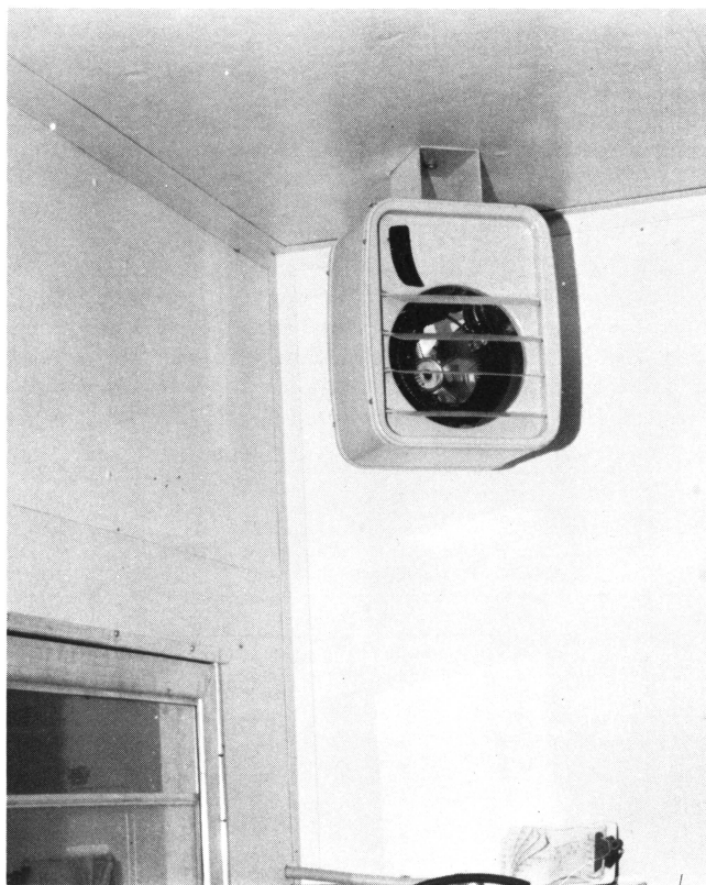
Figure 1. Small thermostat-controlled electric space heater is suspended on the wall in the milk house.
