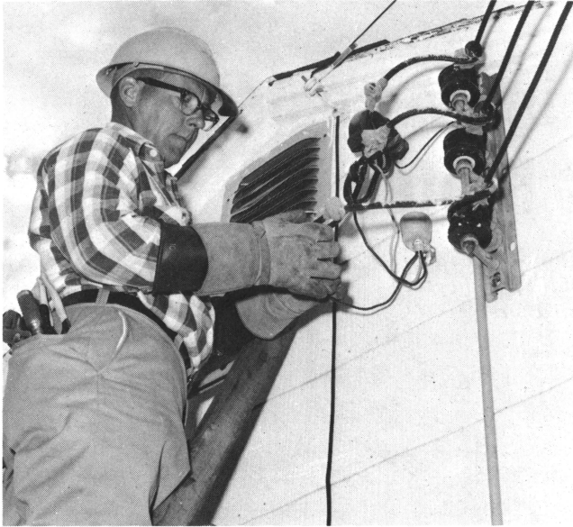
Figure 2. Small lightning arresters, installed by a qualified electrician, provide protection against electrical equipment damage.
