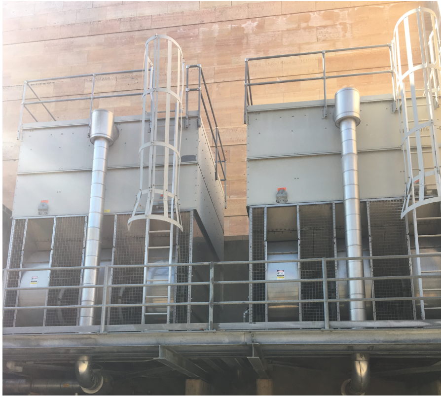
Fig. 3.3.: Eiteljorg's VT-301-0 BAC Cooling Towers
