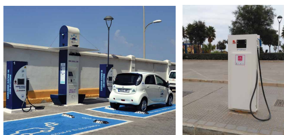
Fig. 33. Fast (left) and V2G (right) charging spots deployed in Zem2all project.
