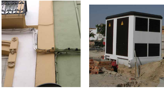
Fig. 3. Facade-mounted, LV aerial bundled cables (left) typically found in towns and medium-sized cities of some European countries, and underground MV cables (right) entering a compact, prefabricated concrete-made secondary substation, customarily used in urban and suburban areas in Europe.
