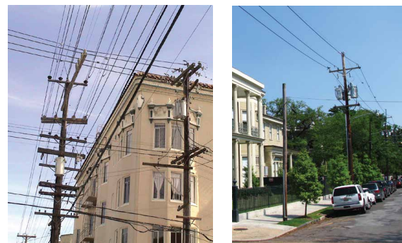
Fig. 2. Urban distribution grids in San Francisco (left) and New Orleans (right), where the same wood pole usually holds both MV and LV feeders.
