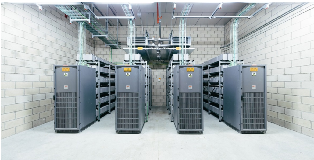
Figure 5.8: Server room in Internet Machine , 2014 (Source: http://www.elasticspace.com ).
