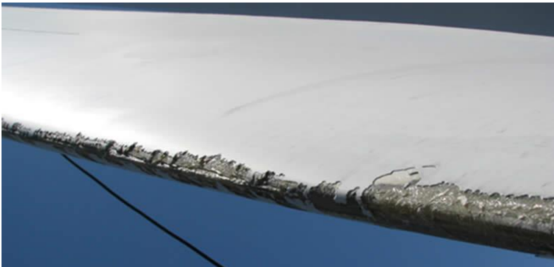
Figure 14: Impact of the erosion on a blade [28]
