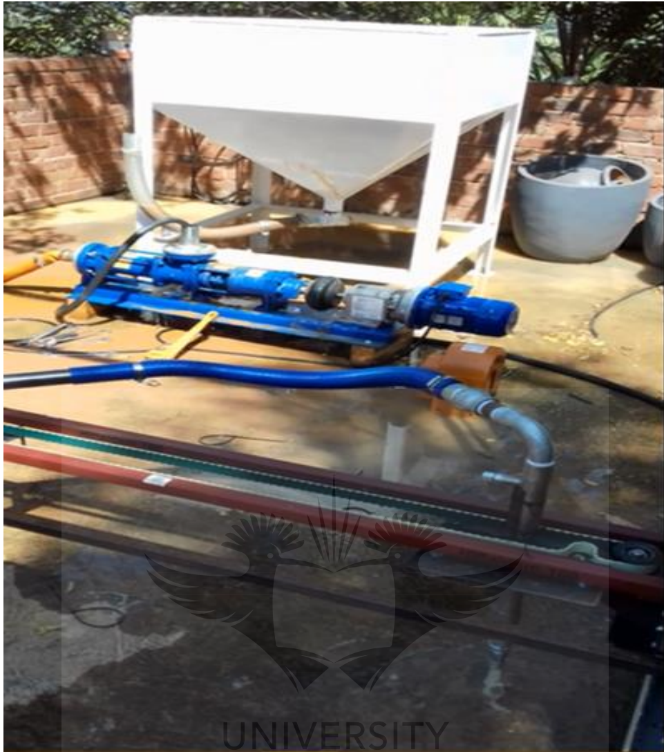
Figure 3.8 Fully integrated system pumping water
