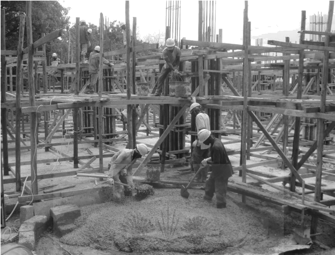
Figure 2.10: Mixing and transporting concrete at a construction site in Dar es Salaam, Tanzania (Msinjili, 2012)
