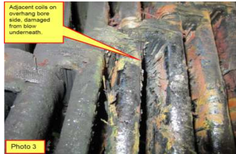
Figure 28: Damage from underneath [63]
