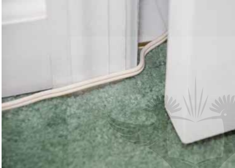
Figure 3 - Example of how line-to-neutral arc fault is created (door pinching power cable)
