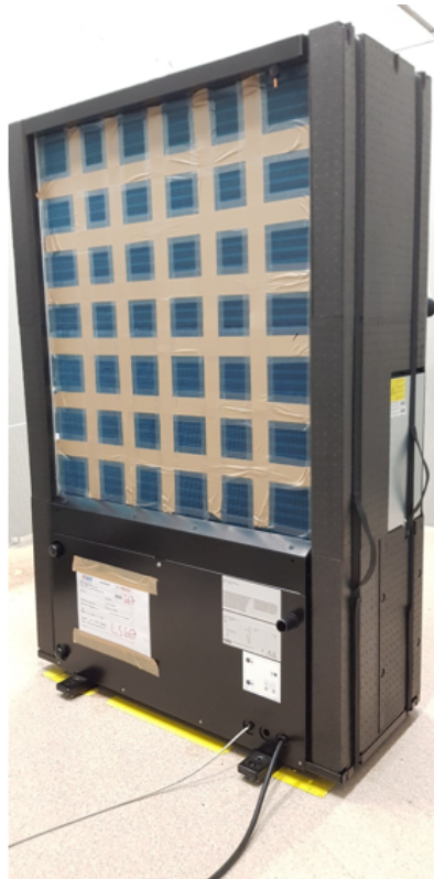
Figure 6.8: Outdoor heat pump fins (inlet) obstructed with tape.
