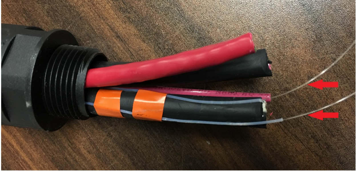
Figure 6 A photograph of the multi-purpose electrical cable fitted with single mode Al-doped and single mode telecommunications fibers (pointed out by red arrows), for real-time monitoring of radiation effects and temperature changes, respectively [49] © 2017 IEEE.
