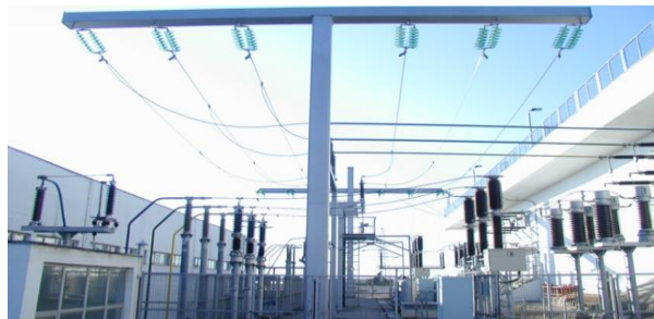
Figure 6. Existing classical 110 kV switchgear
