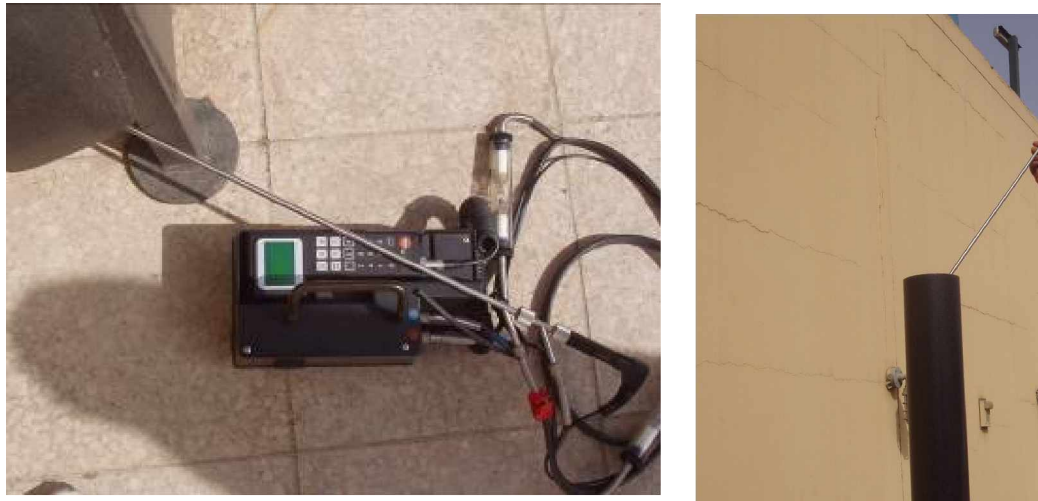
Figure 39: Flue Gas Analyzer and Exhaust Testing
