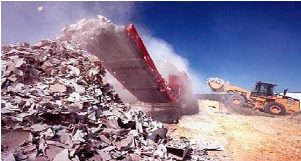
Figure 1.6: Disposal of Waste Gypsum Boards in Landfills (St. Petersburg Times, published, 2000)
