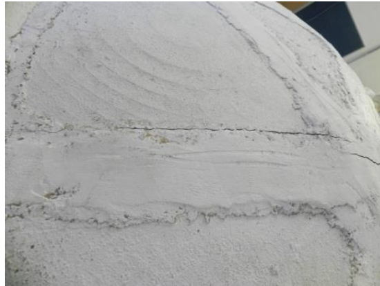
Fig. 179: Cracks at the interface of the panel and the grout at the joint
