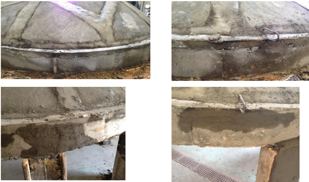
Fig. 104: Ring beam joint cracks
