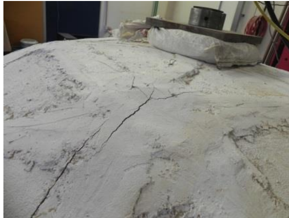
Fig. 180: Meridional cracks at the intermediate joints
