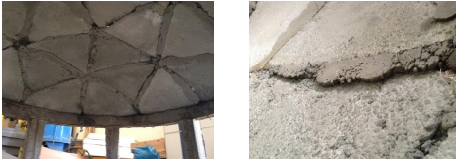
Fig. 105: Superfluous hardened grout on the lower surface of the shell
