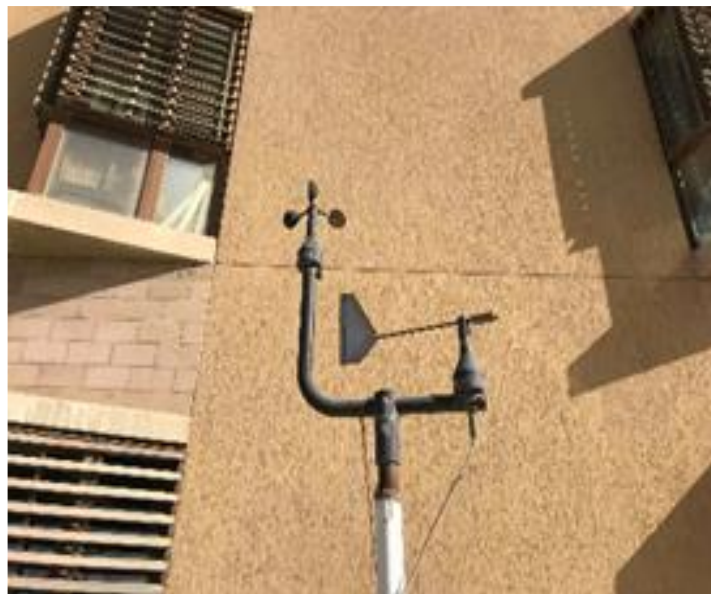
Figure 6-9: A photographic view of the wind speed and direction sensors
