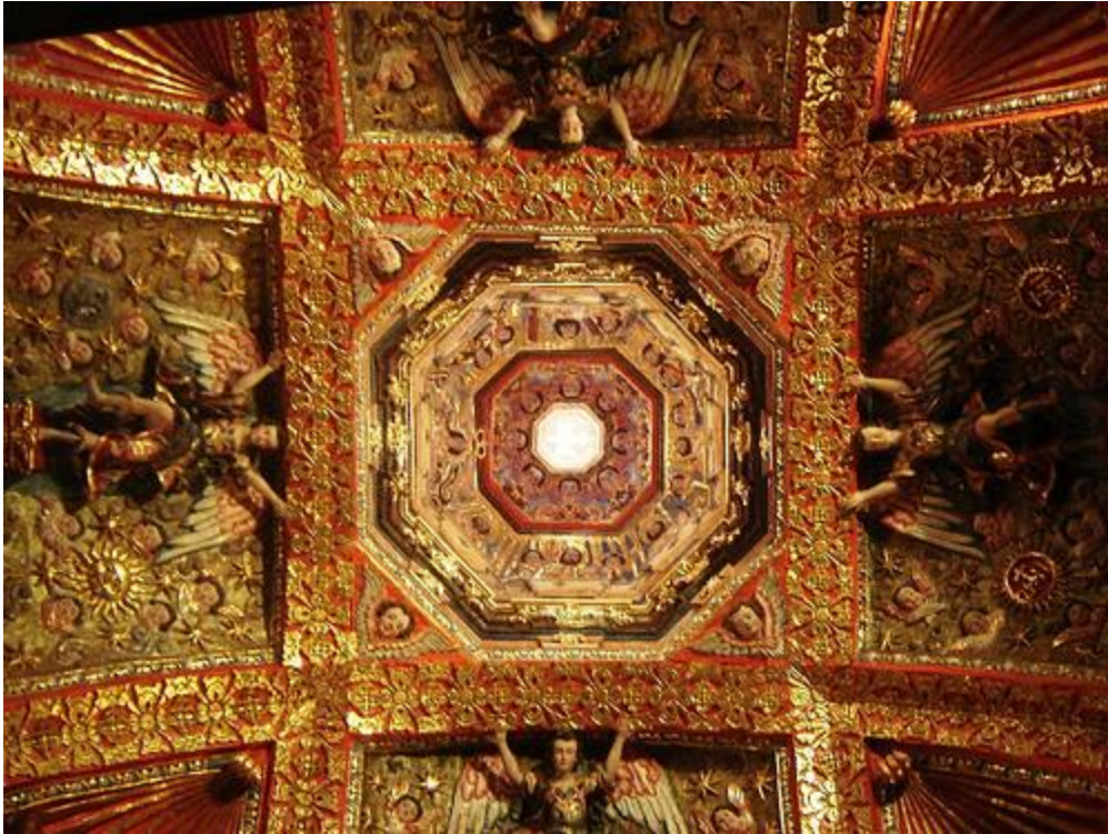
Fig. 1.17 Vault of crossed arches at the Church of Our Lady of Loreto in Tepetzotlan, Mexico.
