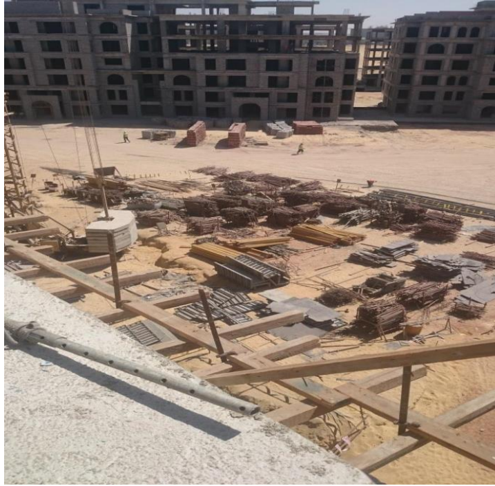
Figure 26: Storing the Commercially available systems on Site
