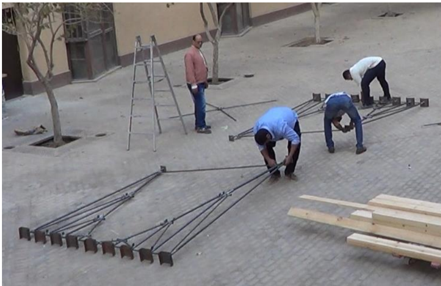
Figure 21: the Tie Rod is connected to the bolts of the bottom chord
