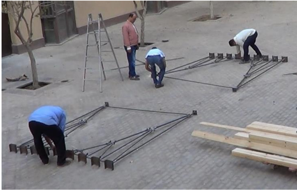
Figure 20: Putting the two halves of the truss in front of each other
