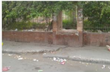
Photo (11) Wrecked pavement with non-standard height
