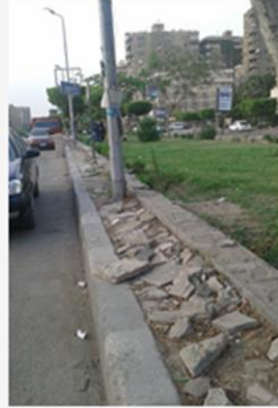
Photo (9) Wrecked pavement
