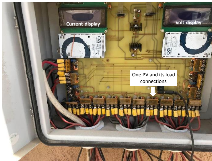
Figure 3-4 PVs data logger with all PVs and Loads connected
