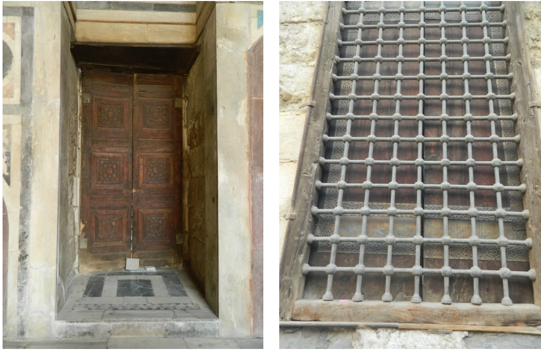
Fig. 35. The windows with wooden shutters in the facade of Sultan al-Zahir Barquq madrasa
