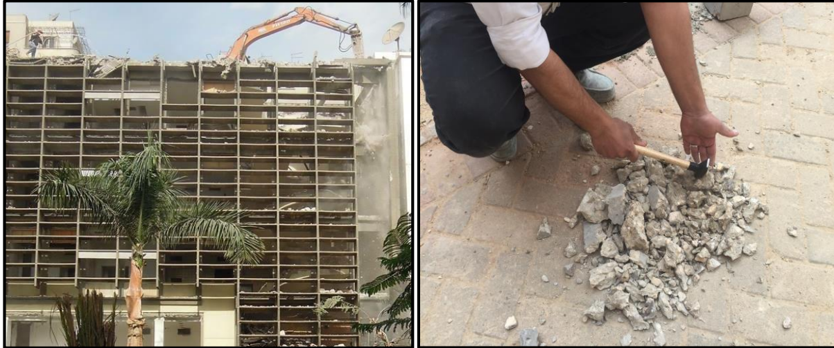
Figure 3-1: Demolishing of Science building of the American University in Cairo Tahrir Campus, October 2015, and crushing the concrete to the desired size.
