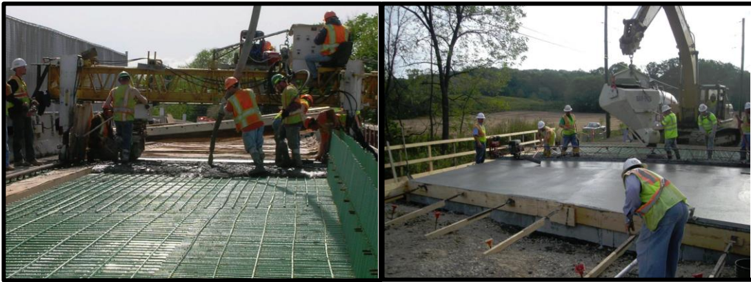
Figure 2-9: Left - Internally cured concrete being cast at Bartell Road in New York (Wolfe, 2010), and Right - Internally cured concrete bridge deck being cast near Bloomington, IN (Di Bella, Schlitter, & Weiss, 2010).
