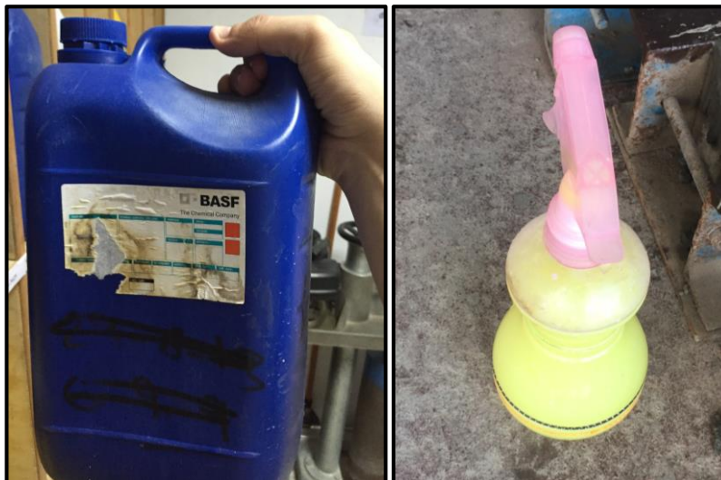
Figure 3-4: BASF MasterCure 181 was used as a curing compound. It was added to a sprayer to be sprayed over the finished surface of concrete
