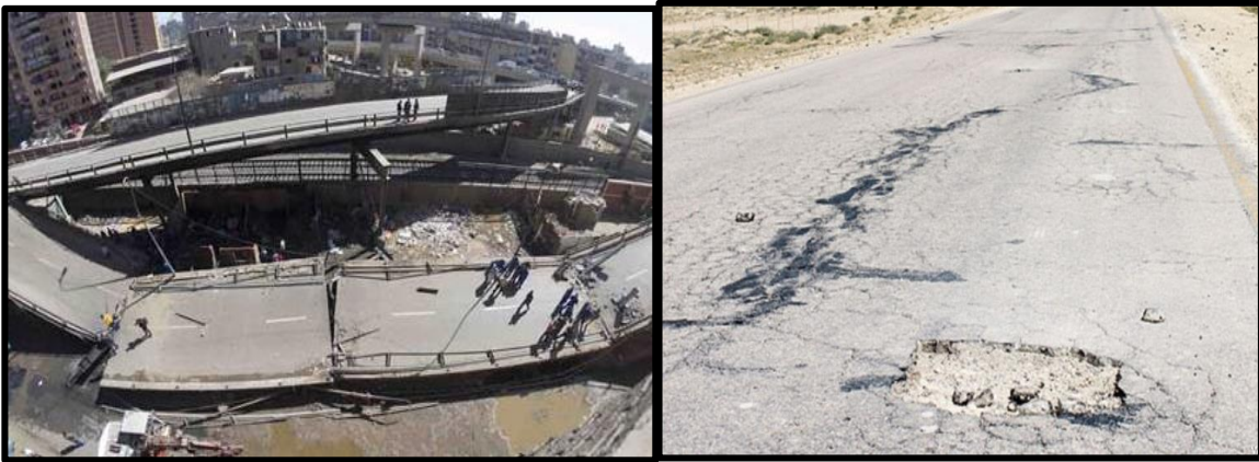
Figure 1-5: Pictures shows the current case of Egypt's Infrastructure, collapsed bridge in Qalyobiya (left) and deteriorated road (right) (Alwafd, 2016)
