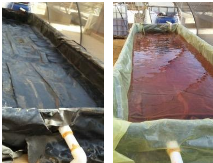
Figure 43: DWC before (on the left) and after (on the right) installing the new vinyl layer.
