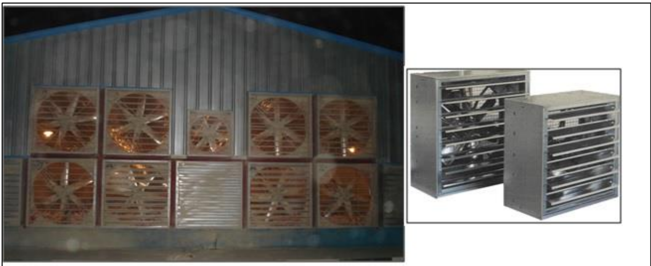
Figure 10: Example of Fans used in Poultry Houses [41]
