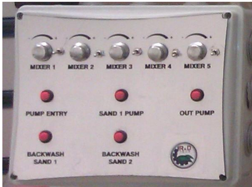
Figure 72: Pumps and Mixer Control Panel
