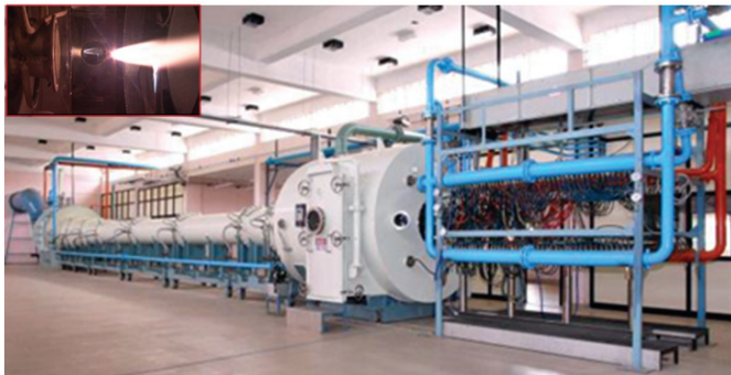
Figure 6. Plasma wind tunnel facility.
