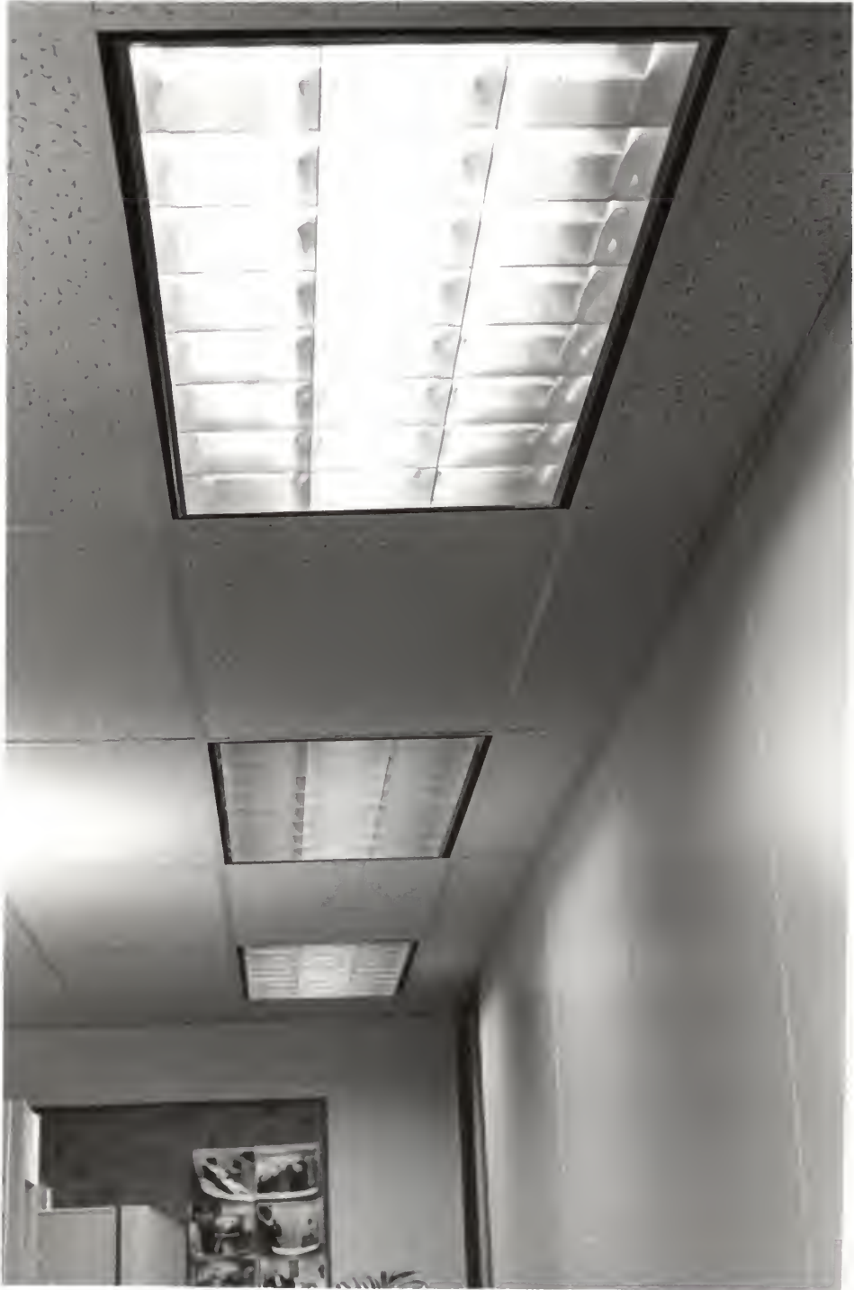
Figure 1. Louvered ceiling lights.
