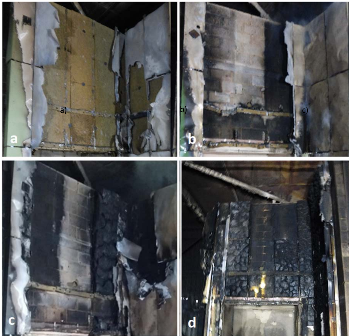
Figure 3 Remains of the tests showing damage around the vent. a) SW/A2, b) PF/A2, c) PIR/A2, d) PIR/PE
