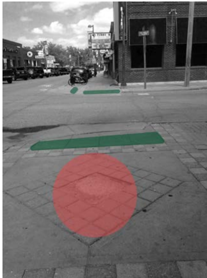
Figure 04: Missing Paver and Tactile Paving
