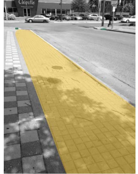
Figure 03: Uneven Side Bricks
