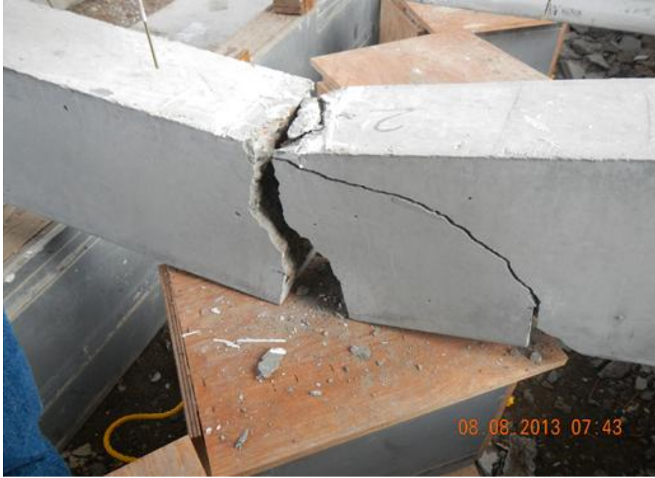
Figure H.77 Beam End G6-L Failure
