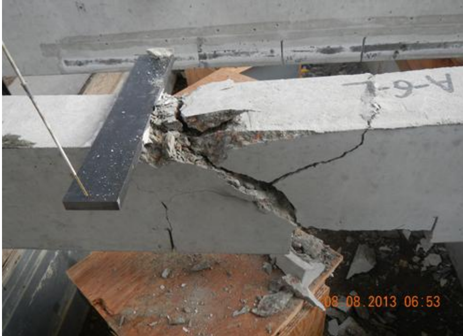
Figure H.18 Beam End A6-L Failure
