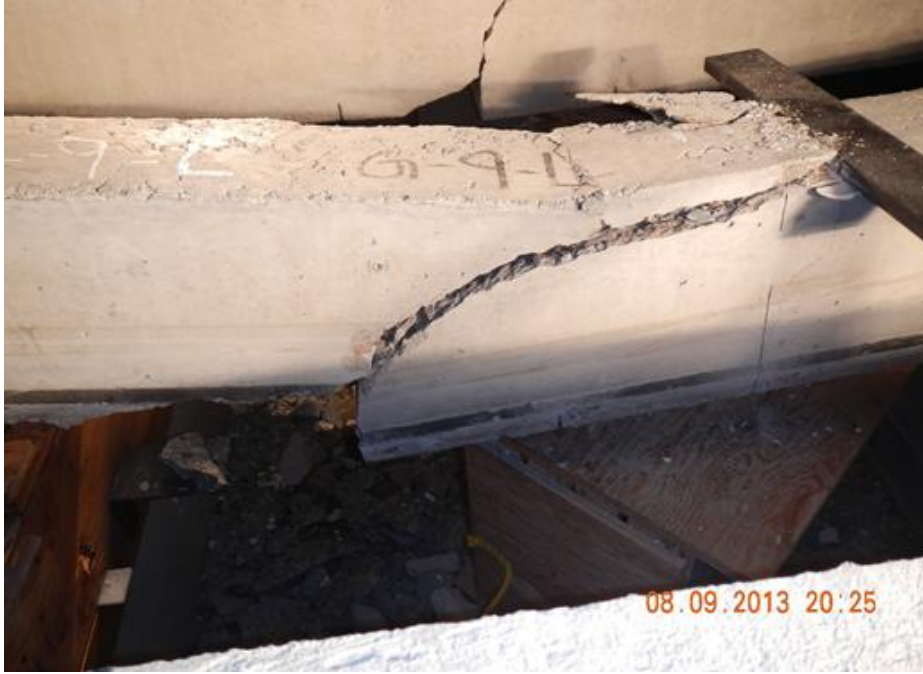
Figure H.86 Beam End G9-L Failure
