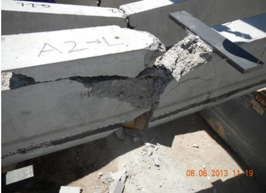
Figure H.6 Beam End A2-L Failure
