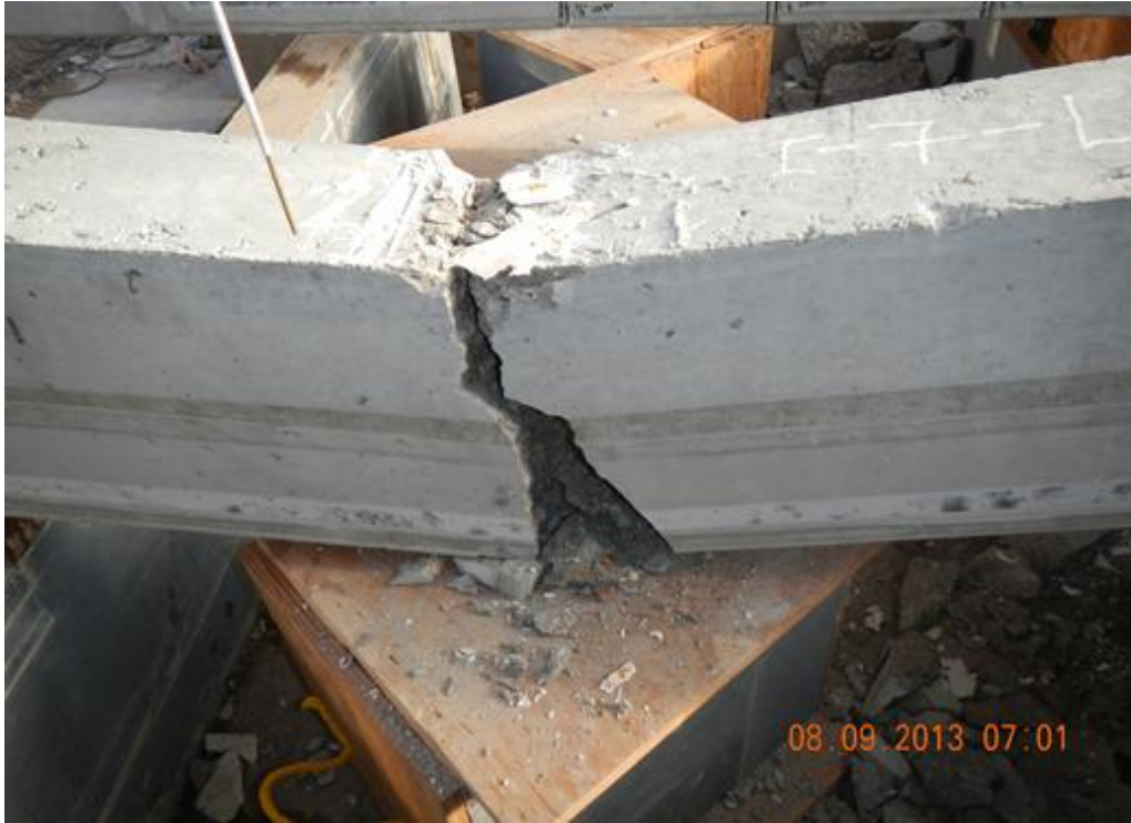
Figure H.140 Beam End I7-L Failure
