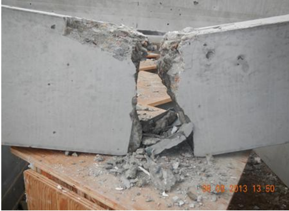
Figure H.164 Beam End I5-S Failure
