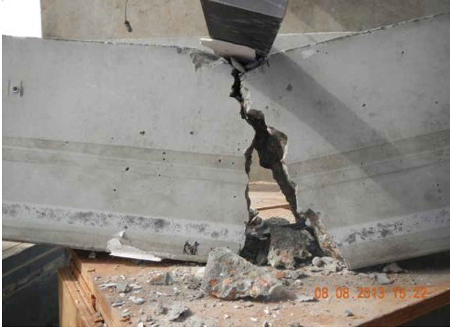
Figure H.137 Beam End I6-L Failure
