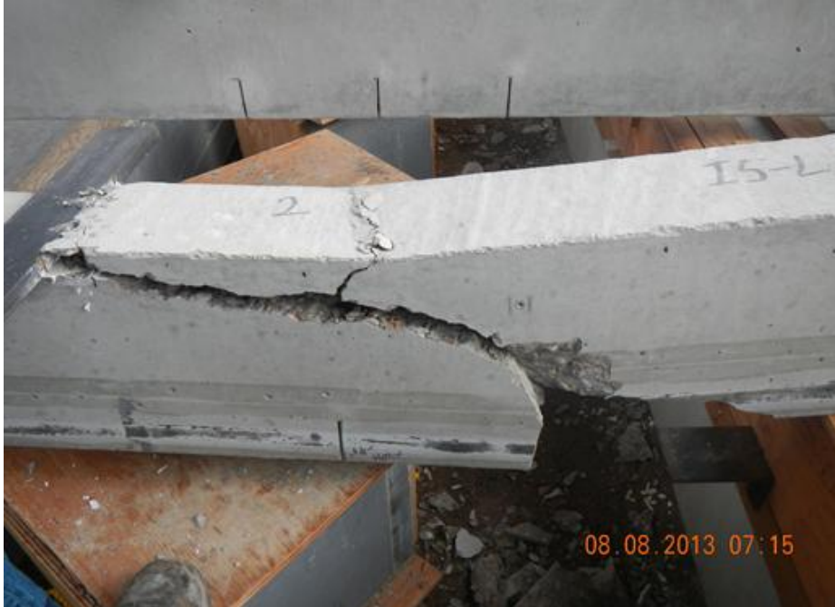
Figure H.134 Beam End I5-L Failure
