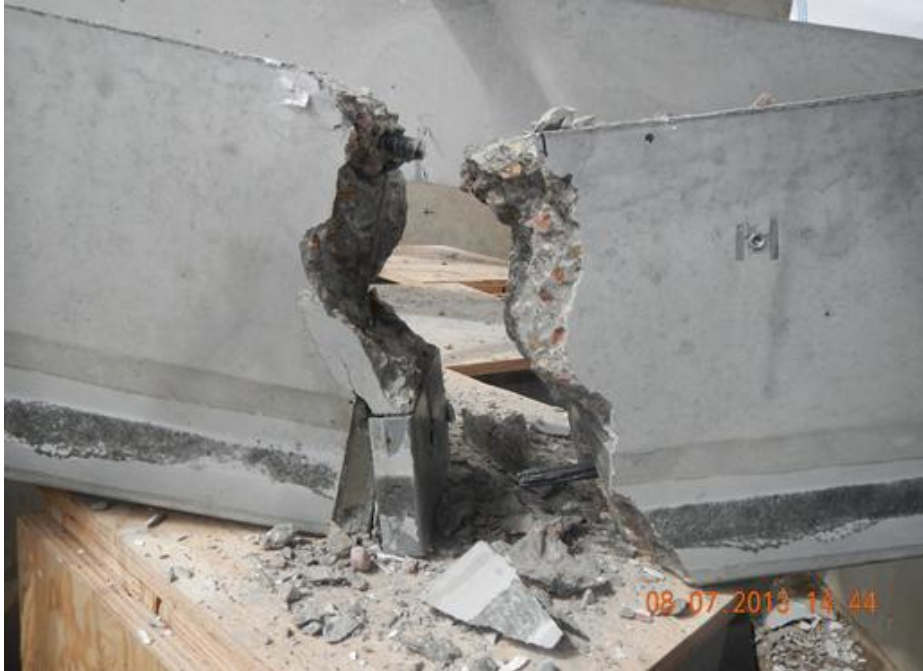
Figure H.42 Beam End A4-S Failure
