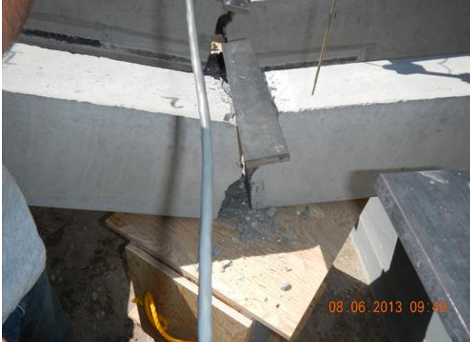
Figure H.122 Beam End I1-L Failure
