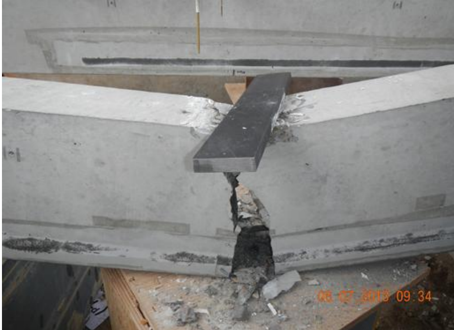
Figure H.131 Beam End I4-L Failure
