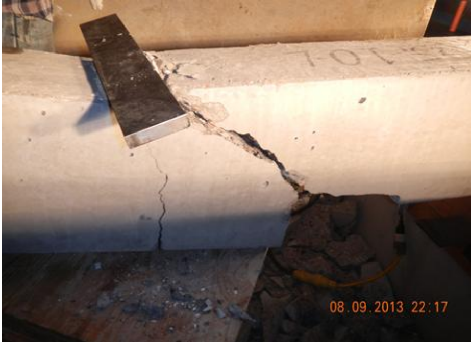
Figure H.89 Beam End G10-L Failure
