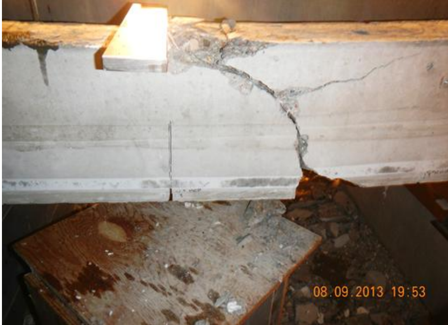
Figure H.146 Beam End I9-L Failure
