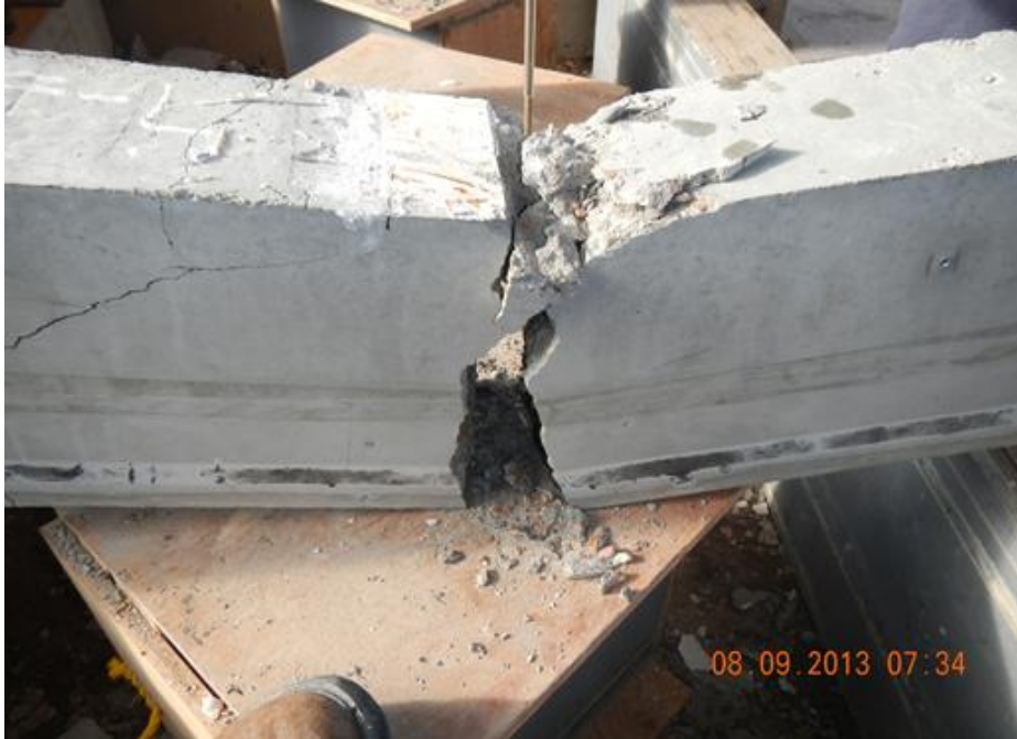
Figure H.80 Beam End G7-L Failure
