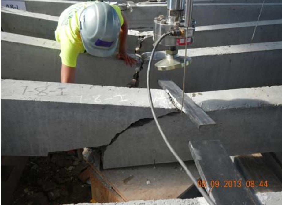
Figure H.143 Beam End I8-L Failure
