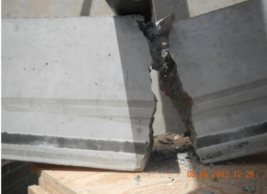
Figure H.65 Beam End G2-L Failure
