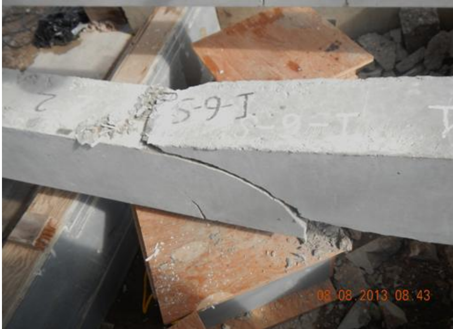
Figure H.167 Beam End I5-S Failure
