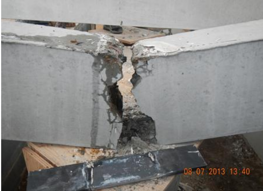
Figure H.158 Beam End I3-S Failure
