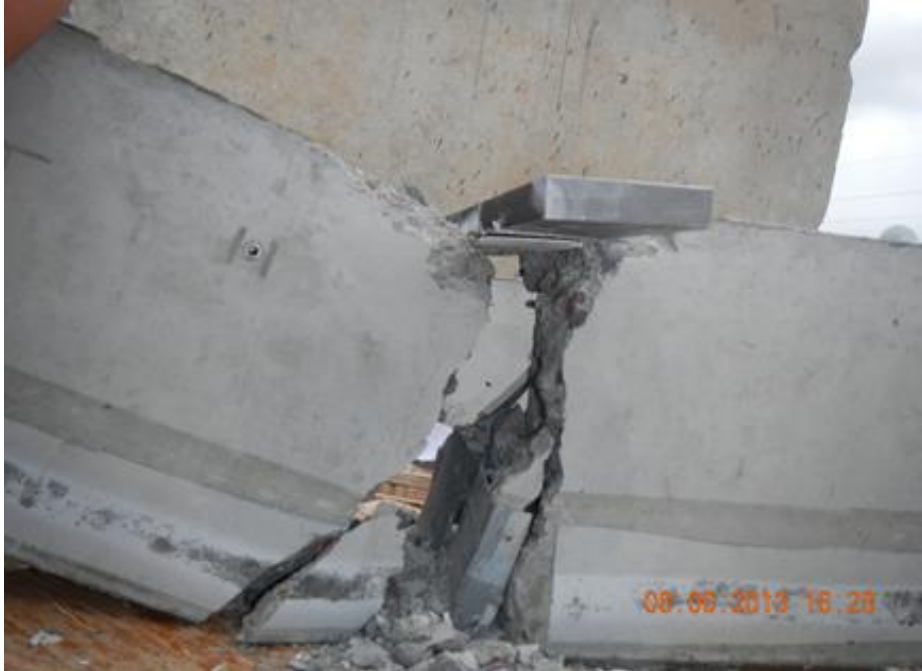
Figure H.152 Beam End I1-S Failure
