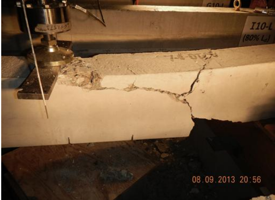
Figure H.149 Beam End I10-L Failure
