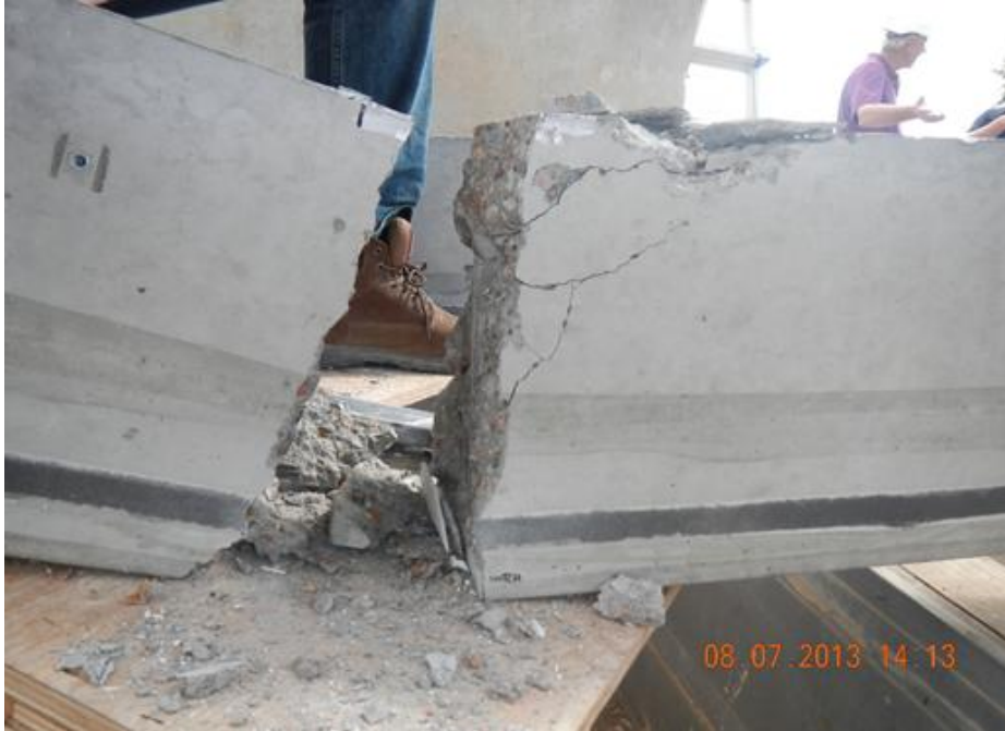
Figure H.98 Beam End G3-S Failure
