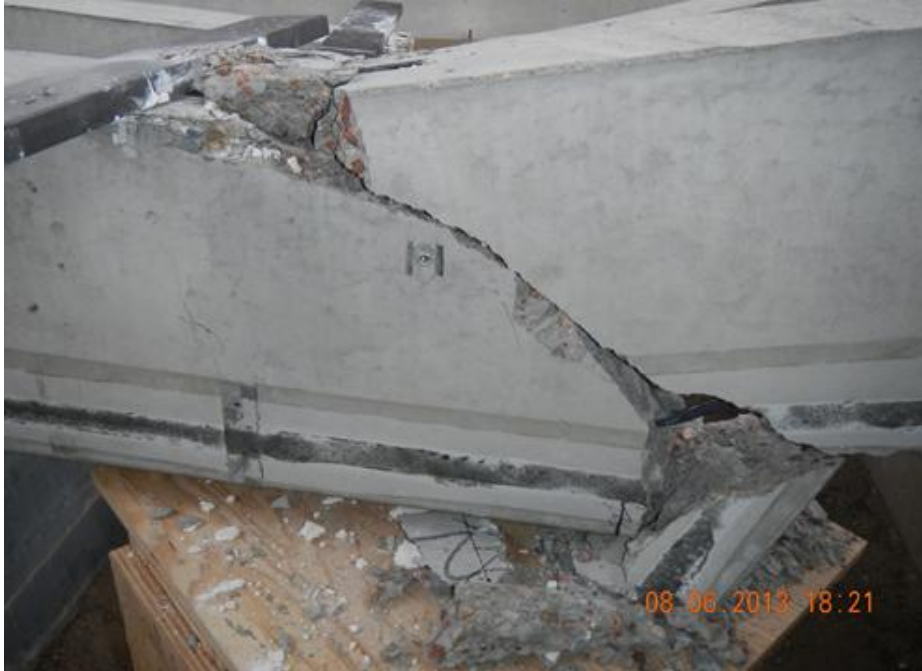
Figure H.36 Beam End A2-S Failure
