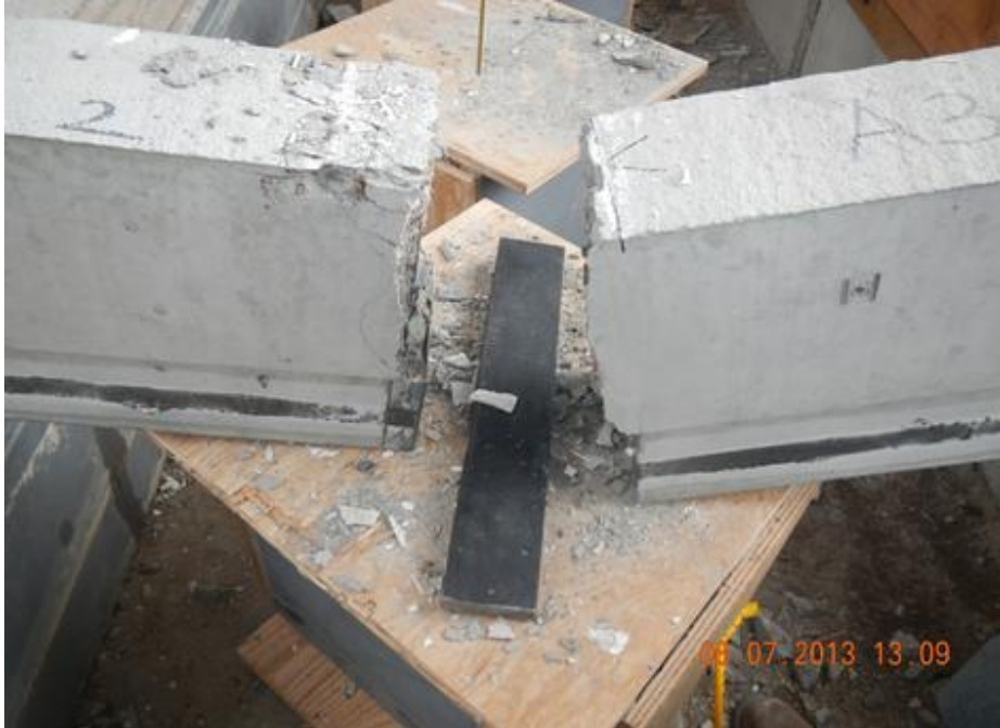
Figure H.39 Beam End A3-S Failure
