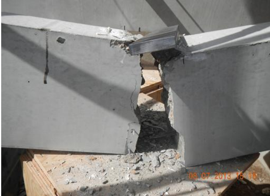
Figure H.161 Beam End I4-S Failure
