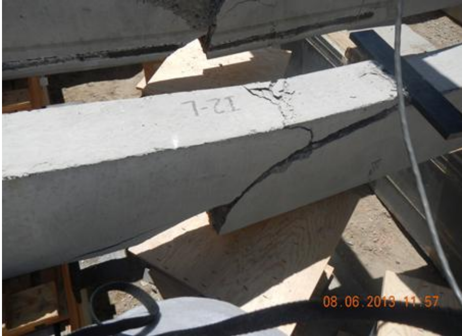
Figure H.125 Beam End I2-L Failure
