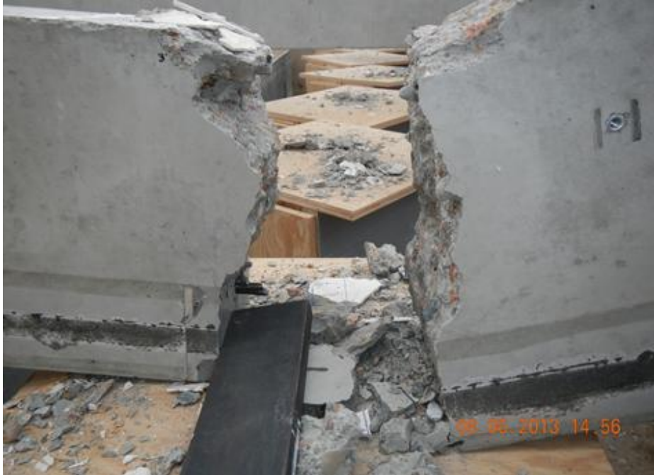
Figure H.33 Beam End A1-S Failure
