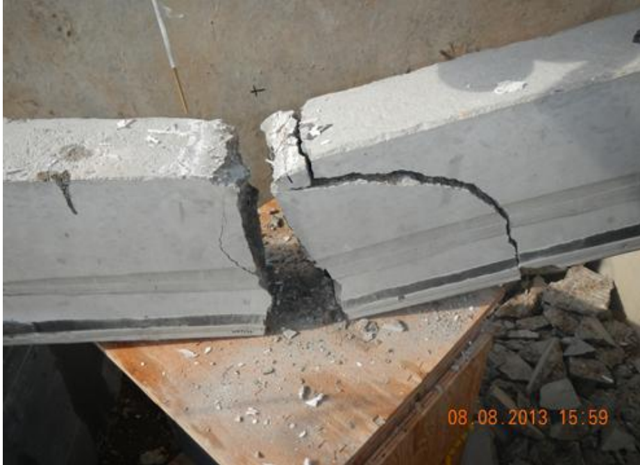
Figure H.74 Beam End G5-L Failure
