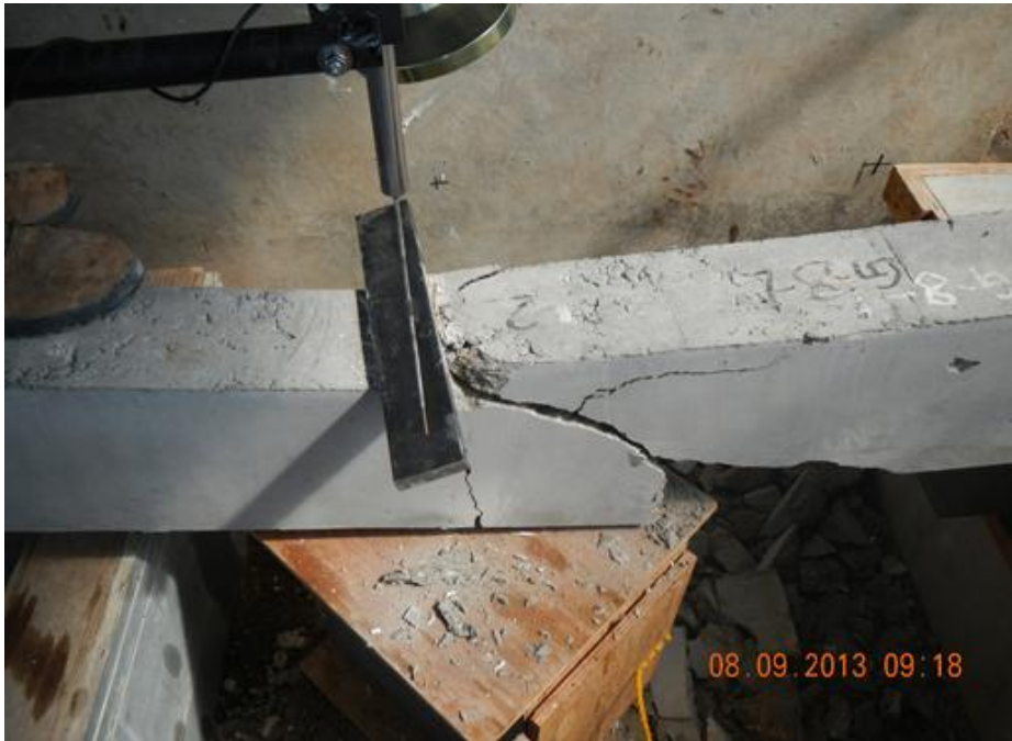
Figure H.83 Beam End G8-L Failure
