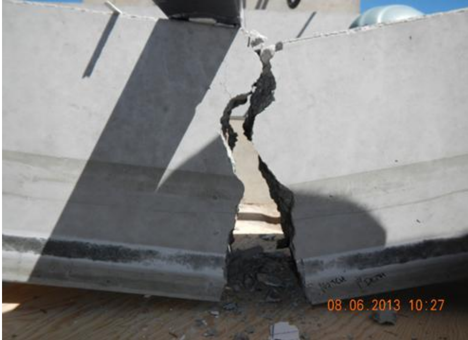
Figure H.62 Beam End G1-L Failure
