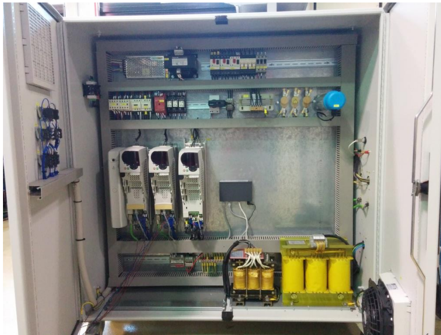
Fig. 5.22. Steel enclosure with the inverters, filters and protections.
