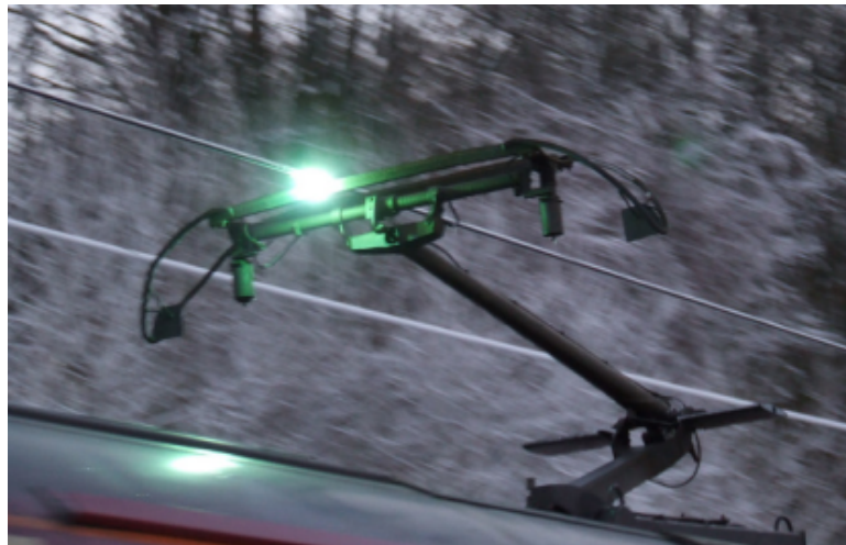
FIGURE 5.2: Arching effect caused by the discontinuity between the pantograph and the catenary.
