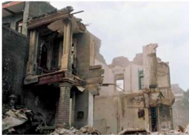
Figures. 97, 98. Zhan Wang, Ruins Cleaning Project , 1994, (top), the artist's cleaning and painting, on the right side of the image, contrast with the next house on the foreground; (bottom), a bulldozer tears down the whole area.
