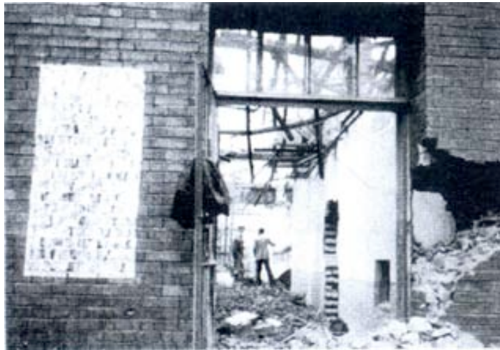
Figure. 92 A photograph showing the rubbing of a wall in a half demolished house in downtown Changchun, 2002.
