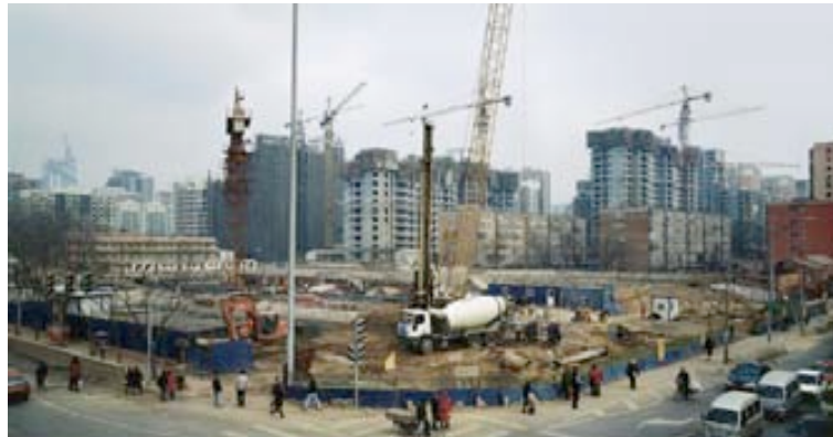
Figures 182, 183. Zeng Li, (top), The construction site of subway line 10, Shuangjing Qiao station, Beijing, 2006 ; (bottom), Chongwenmen Wai Street, 2001 .
