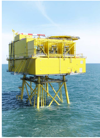
Figure 2.8: BorWin Alpha HVDC offshore platform located in the German North Sea, around 130 km from the coast [77].
