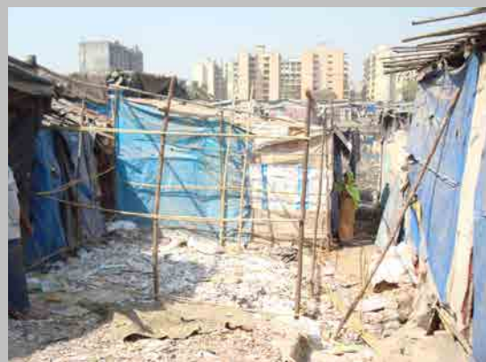
Figure 4.4. First phase of construction of a shelter done by an "informal company".
