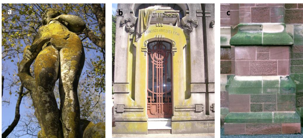
Figure 2.8.- Examples of colonised building materials: a) statue in Portugal, b) portico of a in Argentina and c) detail of a church in Belfast.
