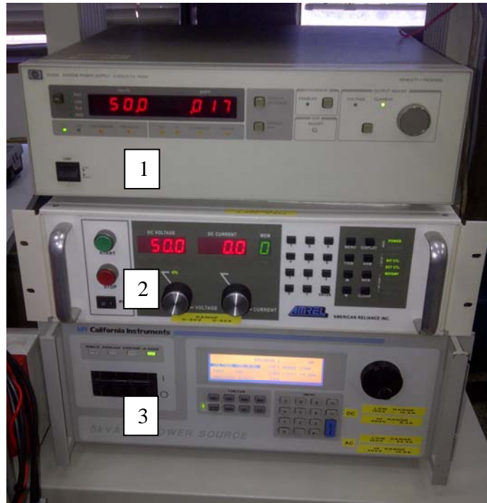
Fig. B.4. DC power supplies.
