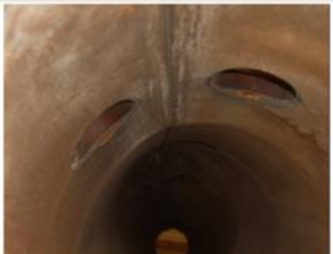
C) Interior of Supply Duct Showing Hose Connector Interface
