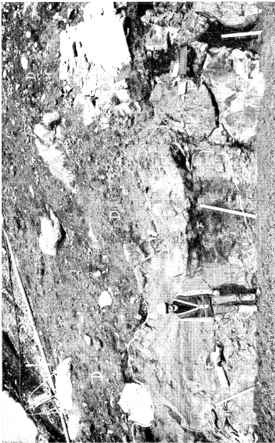
PLATE 2.—A fluvio-glacial sand layer (F) at the base of the glacial drift (D) exposed in the upstream wall of the cut-off trench.
